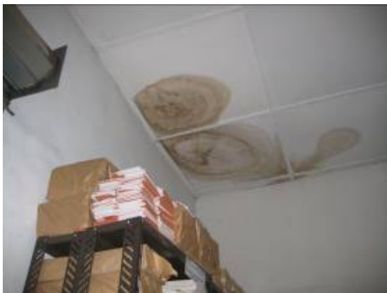
Leakage in the roof, just above a storage area
